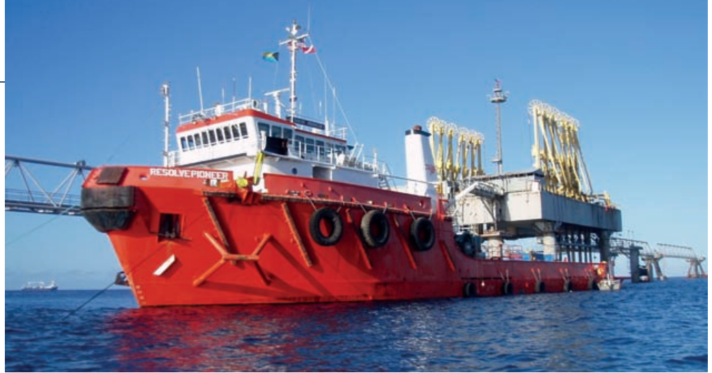
The AHTS RESOLVE PIONEER removing damaged loading platform sections and rebuilding mooring dolphins in Freeport, Bahamas.
